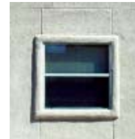
Inappropriate pop-out stucco surrounded by excessive construction joints.
